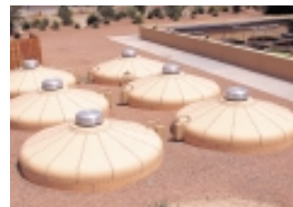
Closed aerobic reactors and operators checking the clarifier
