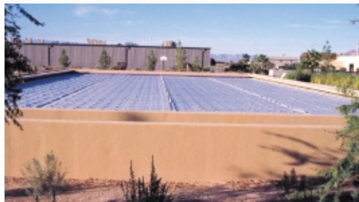
The aerobic reactors, clarifiers and polishing filters are housed within an 8 foot high wall and under a retractable roof which automatically covers the system when it gets cold.
